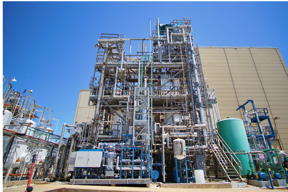
◀ Pilot-scale testing site of the PZ solvent at the University of Texas, Austin. Image courtesy of UT
