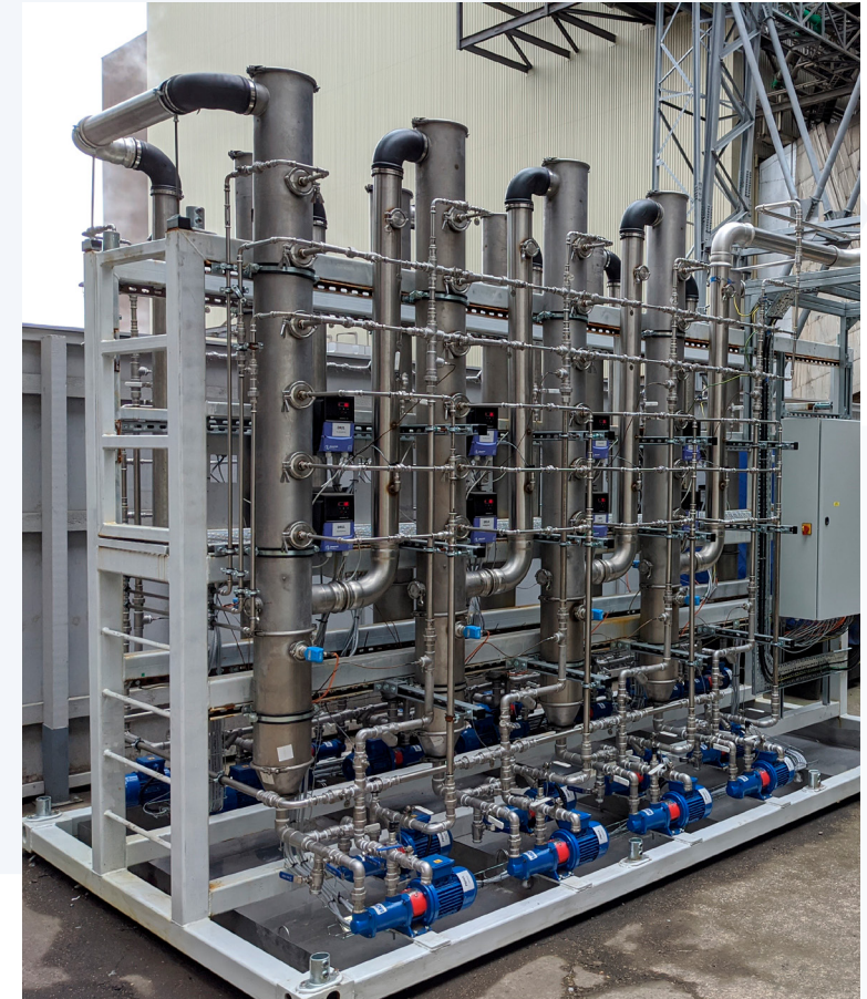
A 10-COLUMN ABSORBER BEING INSTALLED AT DRAX TO IMPROVE THE ABSORPTION RATE OF THE C-CAPTURE SOLVENT IMAGE COURTESY OF C-CAPTURE
