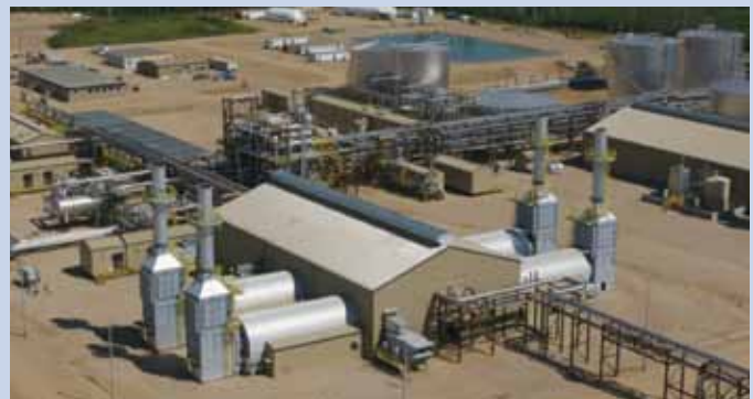
OTSG Boiler. Cenovus Energy, Christina Lake, Canada. Image courtesy of Cenovus Energy
