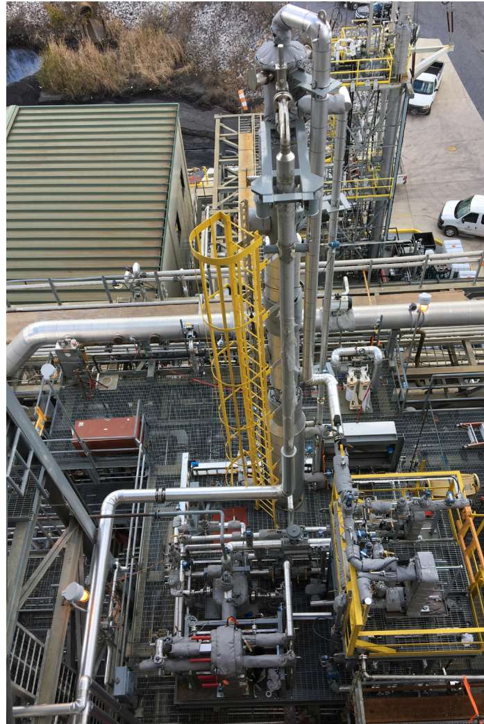
◀ Piperazine technology – advanced flash stripper skid installed at the National Carbon Capture Center (NCCC), Alabama, USA. Image courtesy of UT
