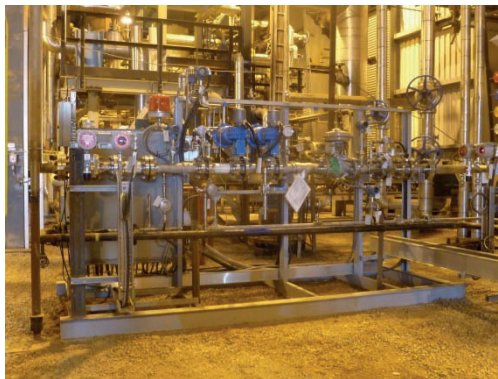
Figure 3. Praxair flow control skid (courtesy of Cenovus and Praxair).
