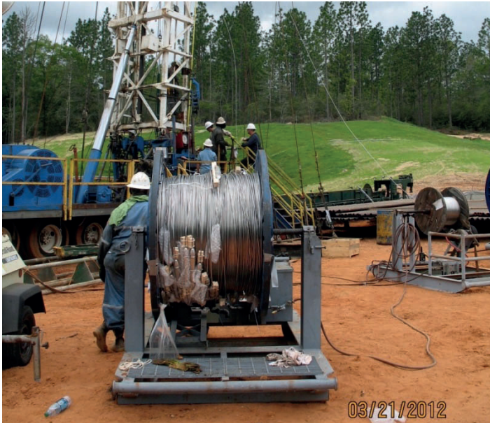
Figure 10. Geophone TEC cable on spool at Citronelle well site.
