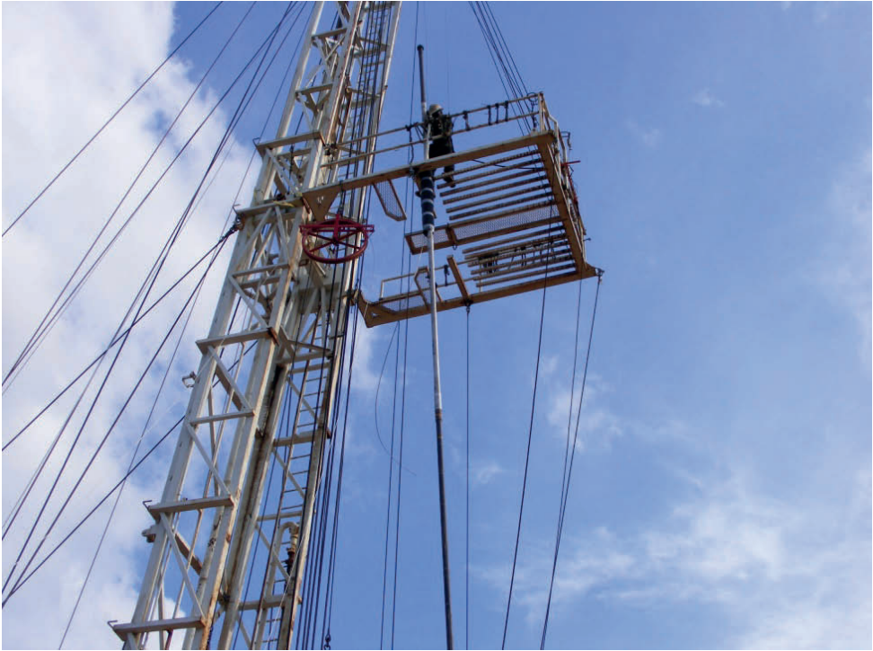
Figure 2. Packer (wrapped in protective cover) and placed vertical in pipe stand prior to starting the run-in-hole of the BHA. The worker has just started feeding the fiber-optic cable through a packer feedthrough and the end can be seen dangling in the air.
