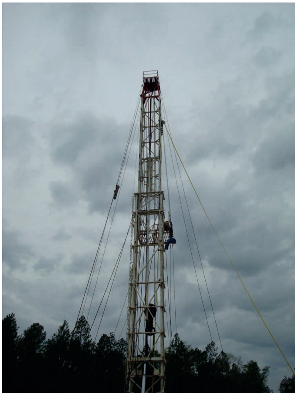
Figure 5. Location of the sheave position high up on the rig derrick for running the flat-pack. The seismic cable sheave was set below the monkey board, but lowered to work-platform height when running geophone pods over the rollers.
