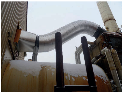
Figure 4. Flue gas recirculation duct (courtesy of Cenovus).
