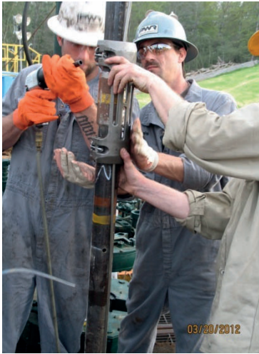
Figure 15. Control line clamp and protector being attached to perforated tubing below packer.
