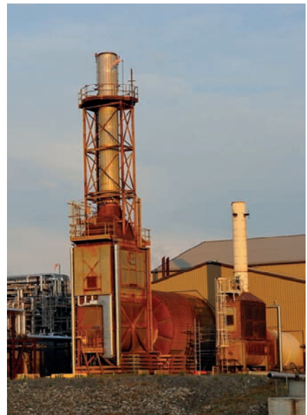
Figure 5. Cenovus Energy Inc., Oxy-fired 50 million BTU per hour Test Boiler.
