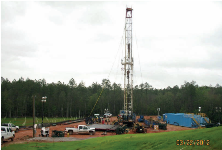
Figure 1. An overview of the worksite showing the placement of the spooling units, pipe stands and mud tanks. Light poles facilitated 24-hour operations.
