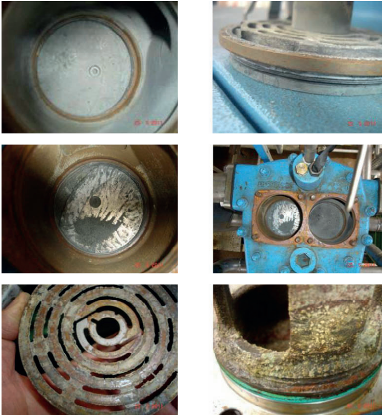
Figure 6. Corrosion inside the recycle compressor.
