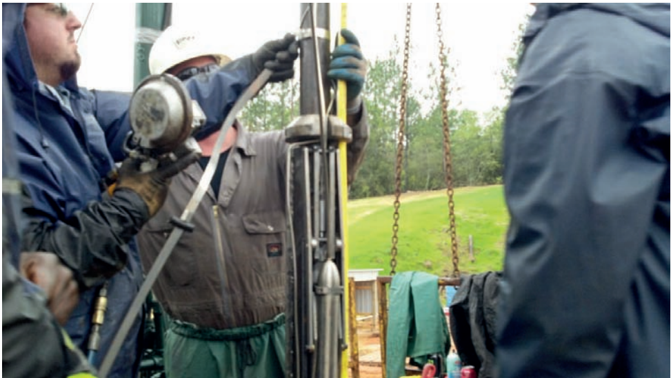
Figure 6. Installing stainless steel bands to organize the cables. Small bands were used at mid-joint locations and above and beneath each geophone pod.
