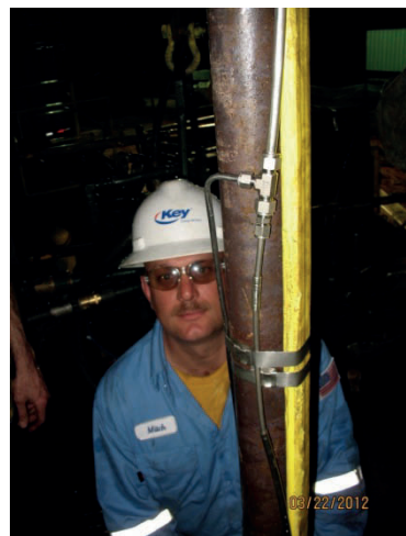
Figure 14. Geophone clamp hydraulic line 'T', along with flatpack attached to production tubing with steel banding.
