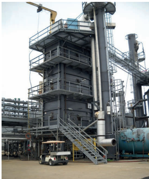
Figure 2. Furnace for oxy-combustion burner tests (courtesy of John Zink Co).
