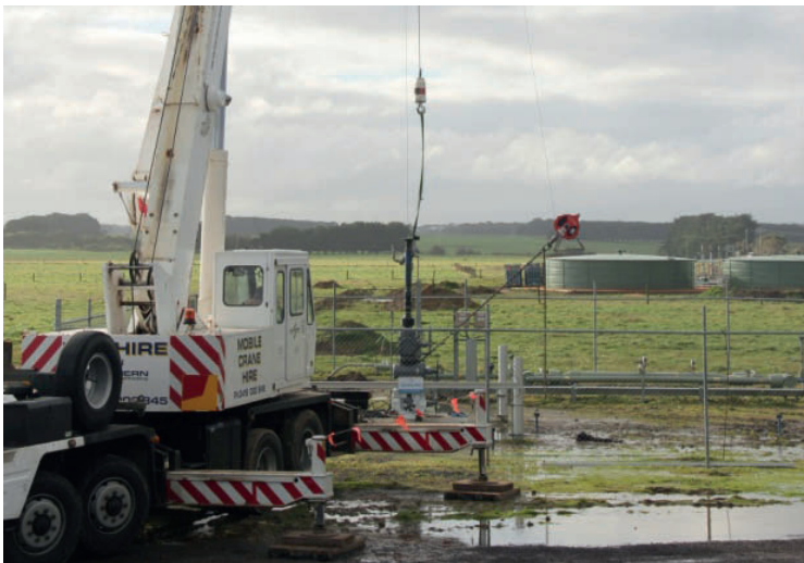
Figure 3. Close up view of the RST logging at the well head.
