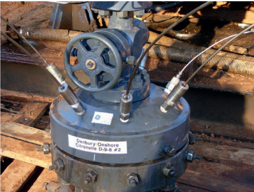
Figure 8. D9-8 wellhead as completed with control lines penetrating through port collars and collar sleeves.
