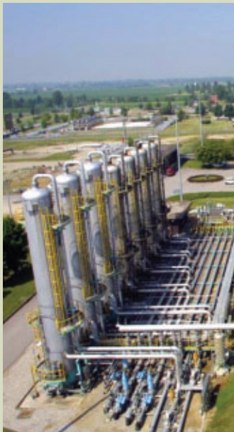
Figure 3.14: Gas storage plant.
