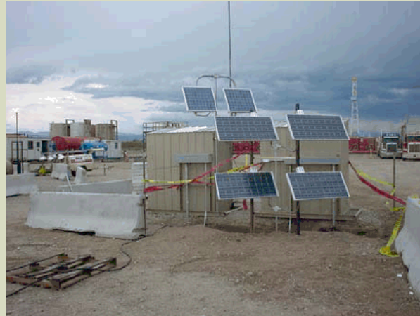
Figure 3.10: Surface facilities for monitoring down-hole pressure and temperature.
