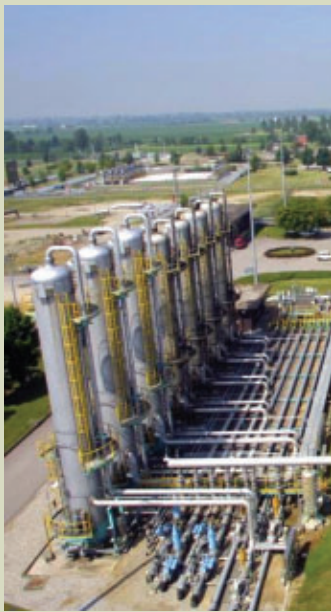
Figure 3.14: Gas storage plant.
