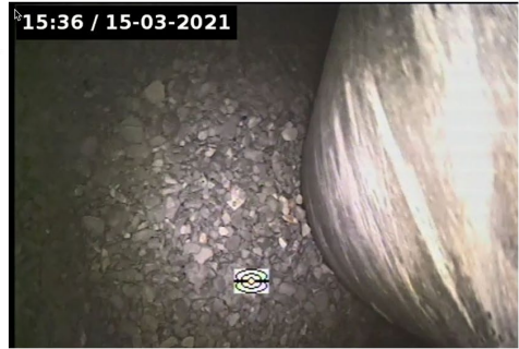
Fig. 8.65m. OPA and cement both have gone at 8.65 m depth (in target section and well below grout packer). Bare 120 mm steel casing of completion is visible on the right-hand side.
