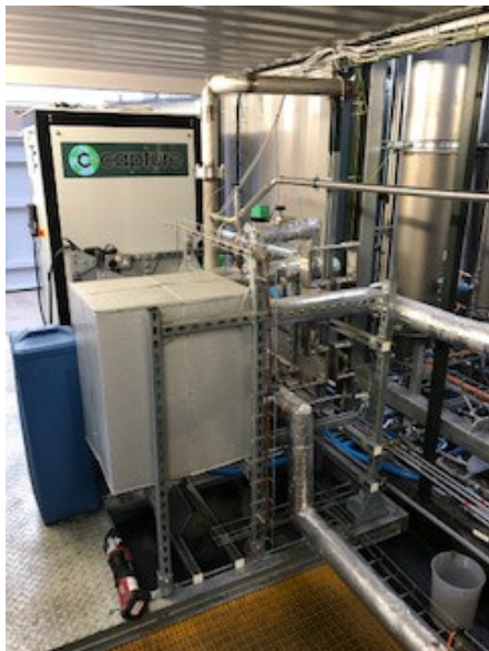
Figure 5. Electric steam generator (at the rear) and reboiler heat exchanger (at the front in an insulated box).
