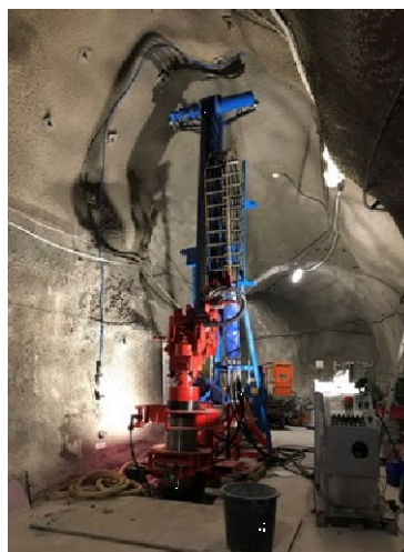
Figure 14. Overcoring drill rig custom-made by SCHÜTZEICHEL GmbH & Co. KG delivered to Mont Terri Rock Laboratory (left) and deployed (right) in Niche EZ-A (Photo: D. Jaeggi, swisstopo).
