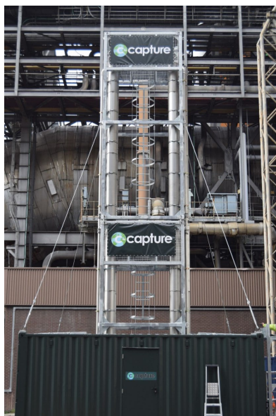
Figure 2. The C-Capture CCS pilot plant installed at Drax.
