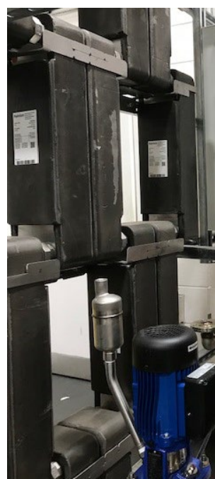
Figure 4. Bank of plate heat exchangers for lean/rich heat integration.
