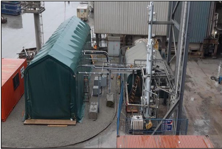
Figure 7. Svante's CO 2 Capture Plant (Phase 1 + Phase 2) at the Lafarge Cement Plant in Richmond, British Columbia.
