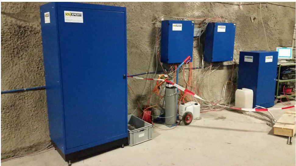
Figure 9. Overview of experimental site with surface equipment (small cabinets are the control boards).
