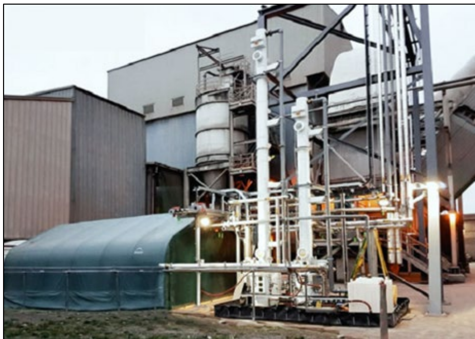
Figure 1. Tri-Mer Pre-Treatment System at the Lafarge Richmond Cement Plant.
