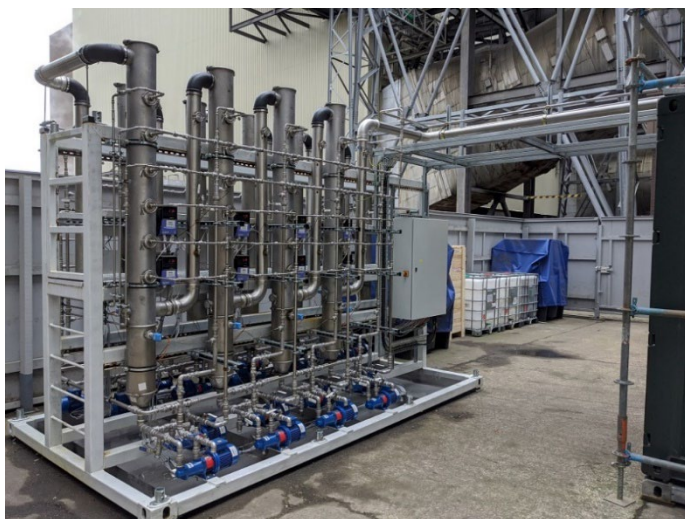
Figure 3. Ten column spray absorber installed at Drax.
