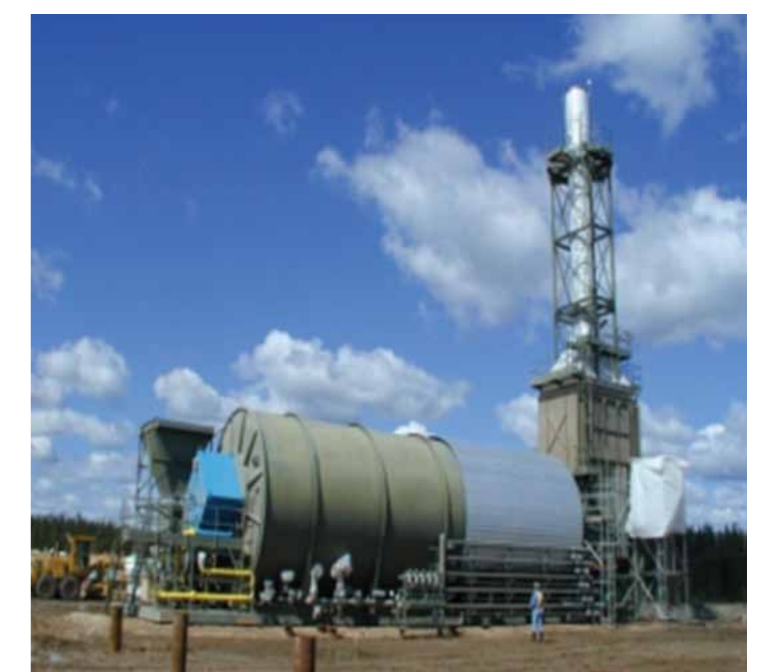
50 million BTU/hr OTSG unit in Christina Lake (Courtesy of Cenovus Energy)
