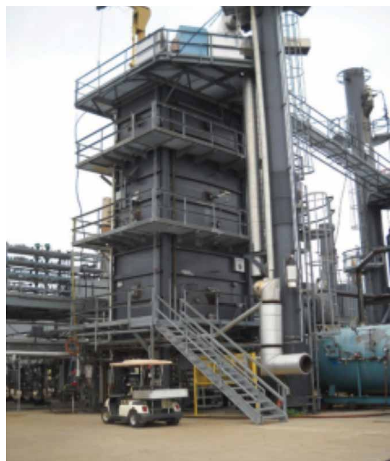
Heater pilot unit in Tulsa (courtesy of John Zink Co.)
