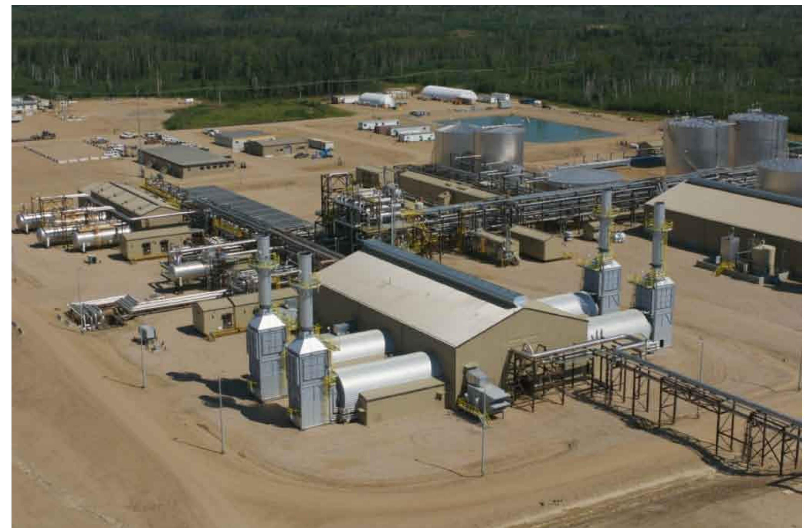
Figure 2 – In-situ Production Site (4 OTSG boilers visible)
