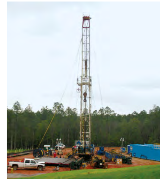
Field trialing of MBM technology carried out in CCP3 at Citronelle Dome, Mississippi, USA. Image courtesy of LNBL
