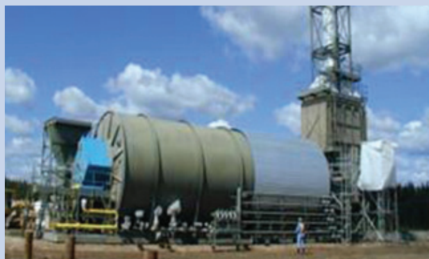
OTSG Boiler. Cenovus Energy, Christina Lake, Canada (image: Cenovus)
